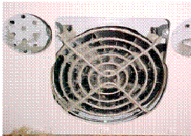
Fig 3. Electric fan controlled by ECS of a industrial machine contaminated by dust and chemical agents
